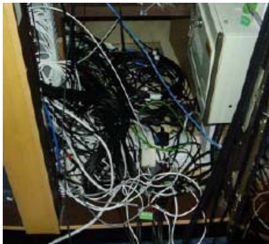
An example of poor quality installation
